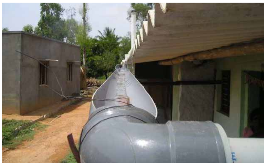
A clean PVC gutter to catch every drop of rain
