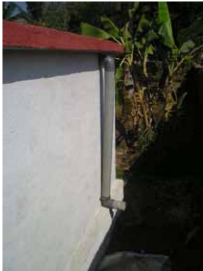
Overflow pipe with mesh
