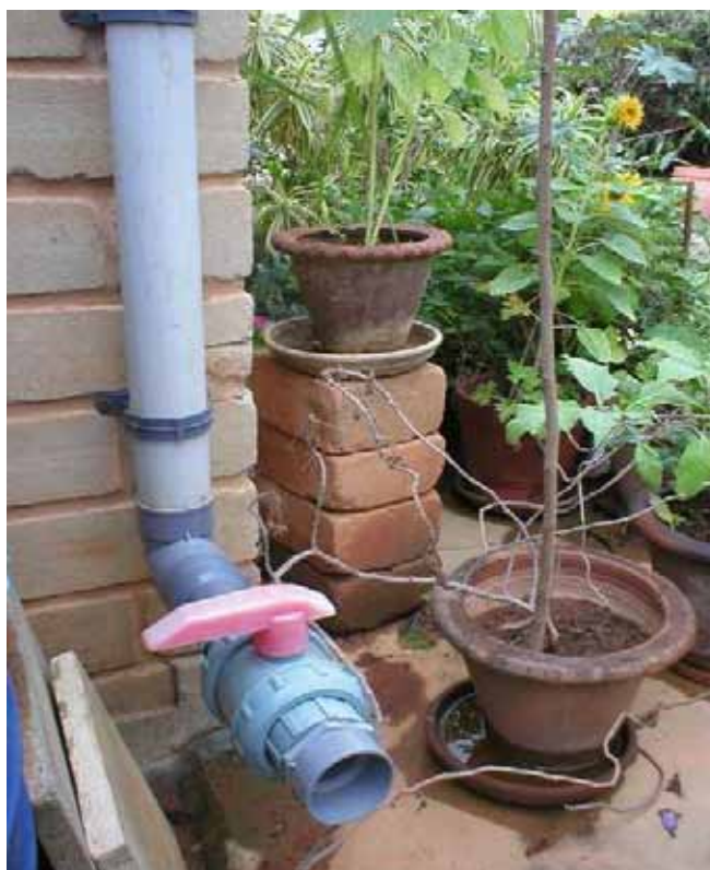
First rain separator with end cap on the wall
