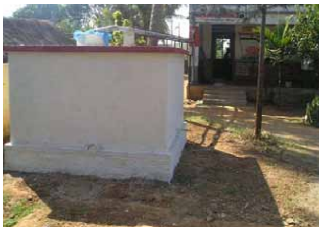
Rainwater storage tank
