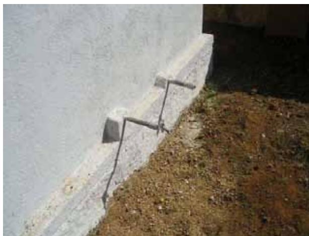
A tap and a drain out pipe firmly anchored to tank
